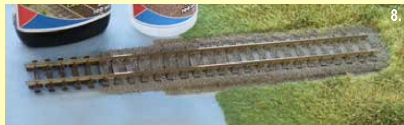
Fig 8. A section of finished track the next day; the Ballast Bond has dried matt ready for action.
