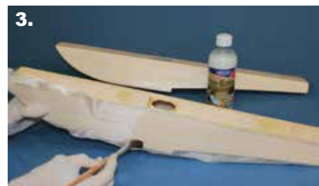
Fig 3. Eze-Kote is then brushed through the glass fabric. The float in the background has already been covered.
